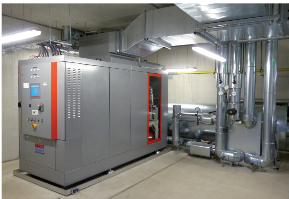
Compact CHP unit GG 198
