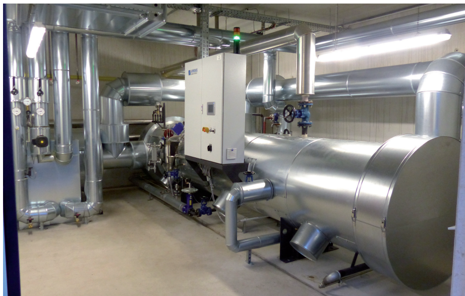
The exhaust heat boiler generates 185 kg/h of saturated steam from the exhaust heat of the cogeneration unit
