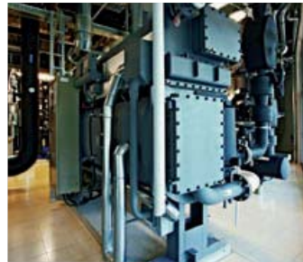
Figs. (from left to right): Daylight use in manufacture, CHP station, Absorption-type refrigerating system
