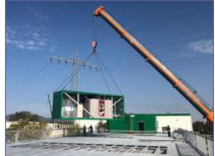
2 Compact CHP units GG 530 H with SCR catalyst, APL Landau
