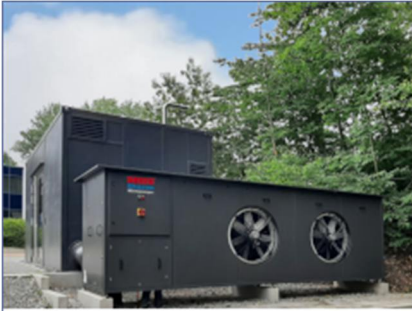
Compact CHP unit GG 50 6VRSB P Air-water heat pump 75 kWth District heating and head office Hiddenhausen
