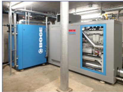
Gas engine compressor unit GK 140 for heat and compressed air generation Heckler & Koch factory, Oberndorf
