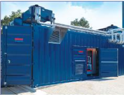
2 Compact CHP units FG 250 Water purification plant Herford
