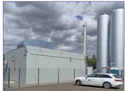
CHP unit GG 1000 District heating in Kitzscher (Saxony)
