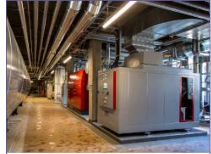
Compact CHP unit GG 260 H Compact CHP unit GG 100 H School and administration center Ravensburg
