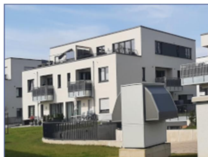
Compact CHP unit GG 50 6VRSB with air/water heat pump Housing on former NAAFI site Herford
