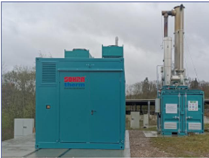
Compact CHP unit FG 95 Landfill Reesberg, Kirchlegem
