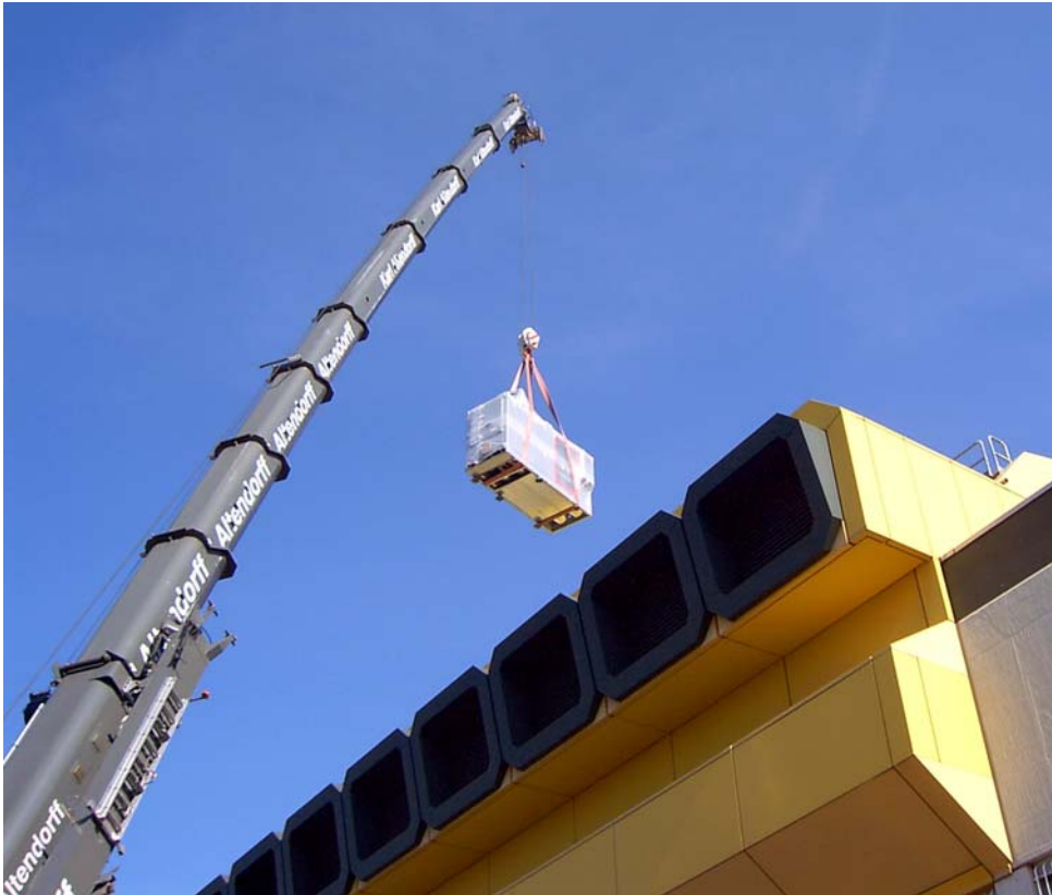
Cogeneration on the rise: Getting the SOKRATHERM GG 383 S into the JVA Berlin-Tegel
